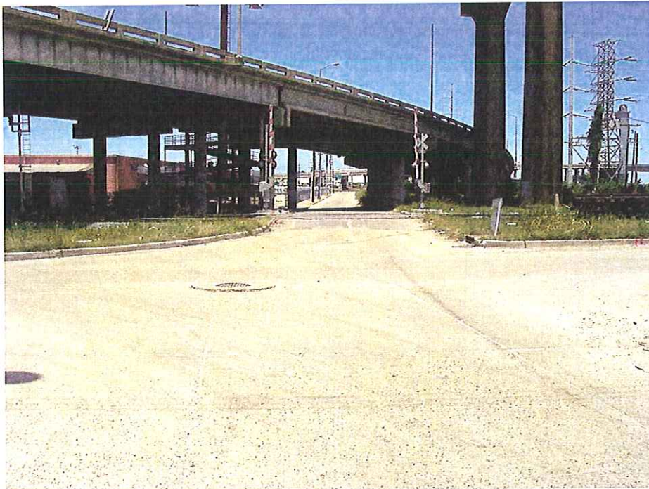
Looking North to Southbound France Road at Almonaster Avenue, Alvar Overpass in Foreground
